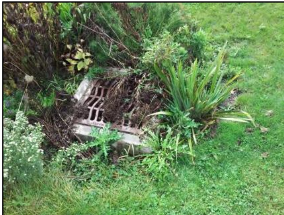
Stormwater flow will be blocked by the dead vegetation on the outlet catch basin grate . Credit: Chagrin River Watershed Partners
