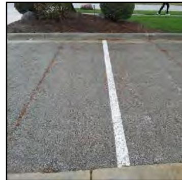
Pervious concrete within a parking lot with debris beginning to accumulate on the surface. Credit: Chagrin River Watershed Partners, Inc.
