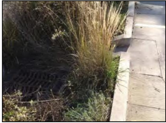
Weeds and untrimmed plantings prevent stormwater runoff from entering the bioretention area from the curb cut. Credit: Northeast Ohio Regional Sewer District
