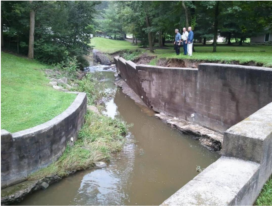
Figure 8: Another example of a costly hard-arming structure used to prevent erosion that ultimately increased erosion.
