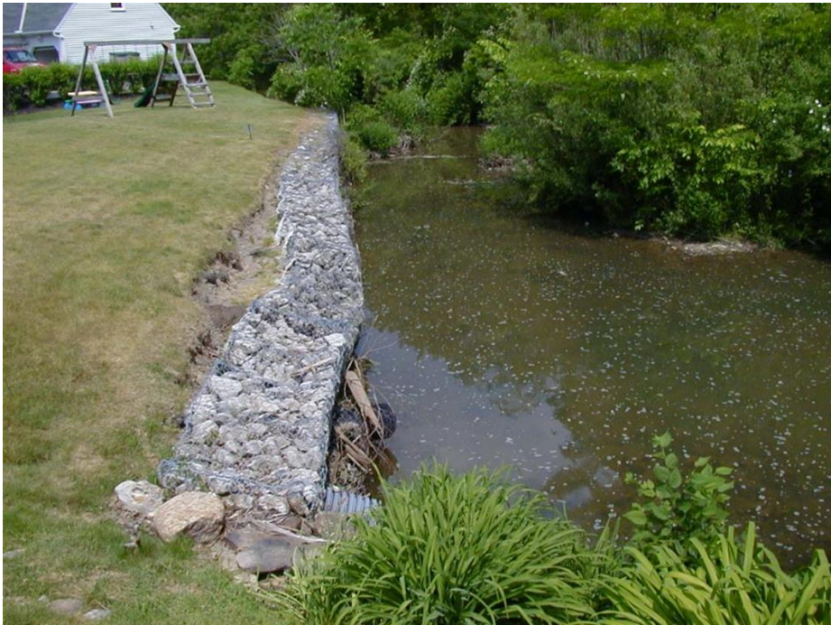
Figure 7: Gabion baskets (pictured) and other hard-armoring solutions are sometimes used to address eroding streambanks, but these solutions are costly and prone to failure. The best solution would have been to site the home further away and not clear land up to the stream. Photo source: Chagrin River Watershed Partners.
