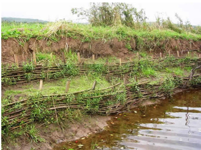
Fascines are live branches that are bound together in long tubular bundles, then placed in shallow trenches across the slope of the streambank.
