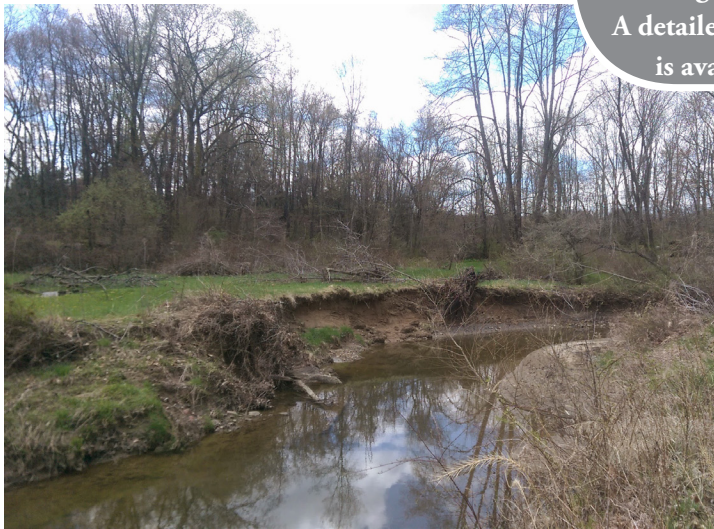
Figure 1. Example Streambank Exhibiting High - Very High Erosional Potential (<50% streambank protection, overhanging roots, <50% vegetation)
