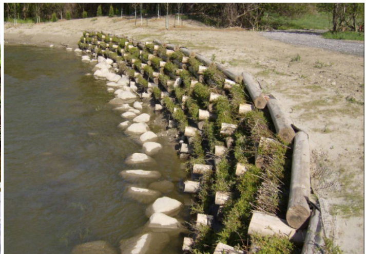
Cribwalls are wooden log cabin-type structures built into the streambank and filled with rock, soil and willow cuttings.
